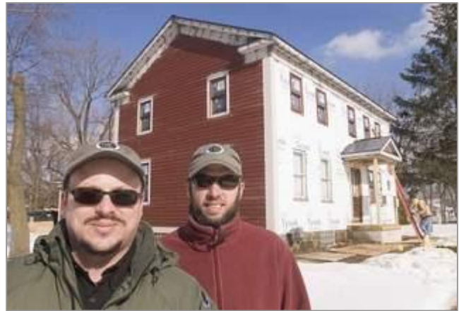
Brian Halprin and Brad Lavey of Green Building Services oversaw the green renovation of the house
